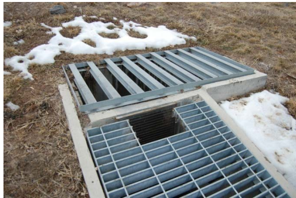
Photograph OS-4. Maintenance access to the water quality trash rack was compromised by the location of a secondary trash rack on this outlet. This may have been included as a safety rack or as additional protection from clogging. The owner modified the structure for better access. A safety rail would have been a better solution.
