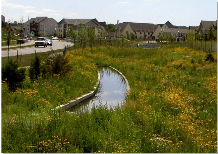
Photograph GB-3. This level spreader includes the added benefit of a sedimentation basin prior to even distribution of concentrated flows from the roadway into the grass buffer. Photo courtesy of Bill Wenk.
