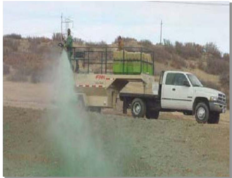
Photograph SB-1. Tackifier being applied to provide temporary soil stabilization. Photo courtesy of Douglas County.
