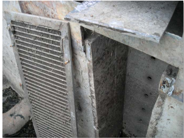
Photograph OS-2. This trash rack could not be properly attached due to its inadequate flange width.
