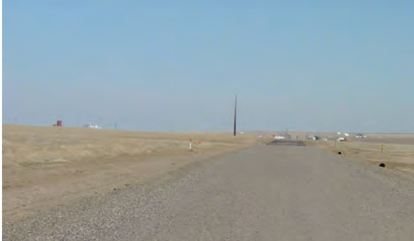
Figure 24: Unpaved Section of Imboden Road
